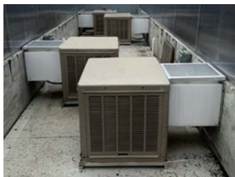
External Evaporative Coolers
